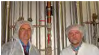
Vulcan installed in a food factory
