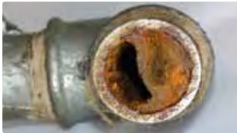
Pipe with scale deposits
